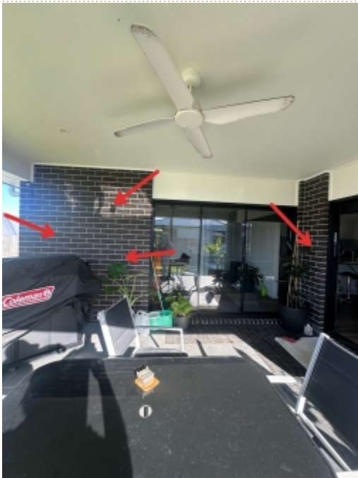
Photo(s) of Defect
