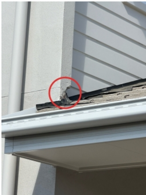
Details of Major Defect
